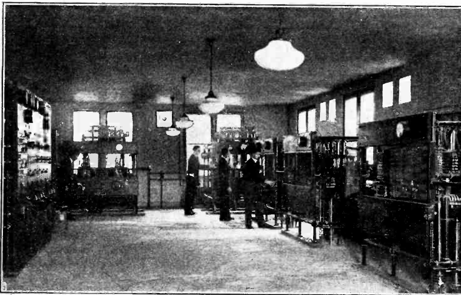
AN AMERICAN HIGH-POWER STATION. America's ambitions in broadcasting are indicated by the construction of WJZ, Bound Brook, N.J., operating with a power of 50 kW. The above photograph was taken in the transmitting room, which actually contains three 50 kW instruments, including an emergency transmitter and a short-wave set.
